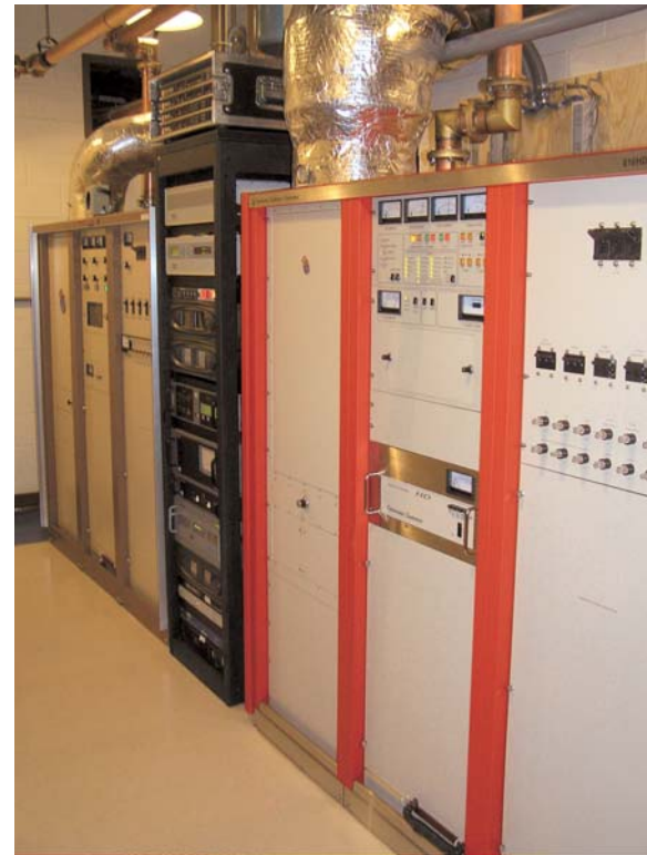
KRQQ's 816HD transmitter alongside the 816R-3 (now the Backup).
