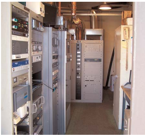
A tightly packed transmitter room.
